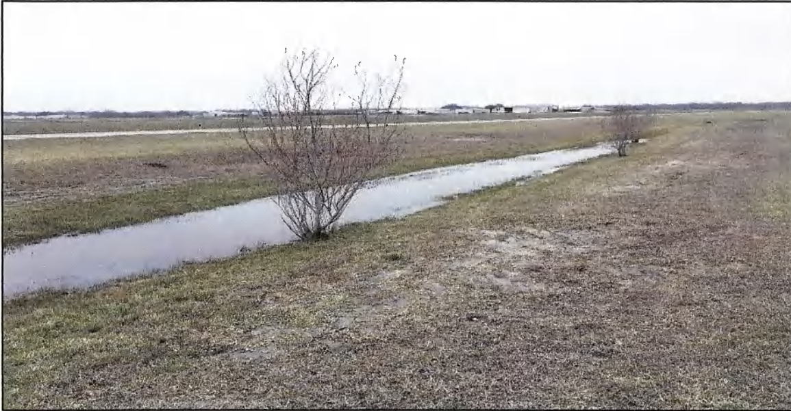
Figure 2. Ponding water in the existing ponds and ditches.
