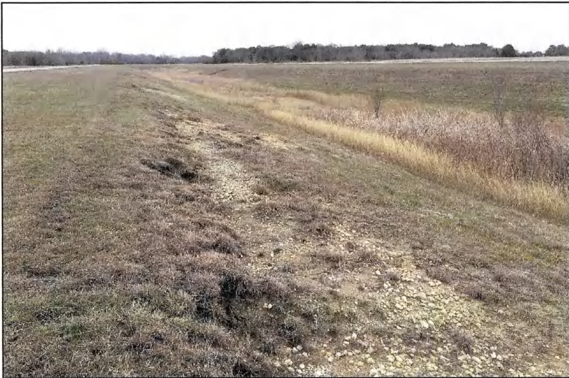
Figure 1. Erosion of the banks of the existing detention ponds.
