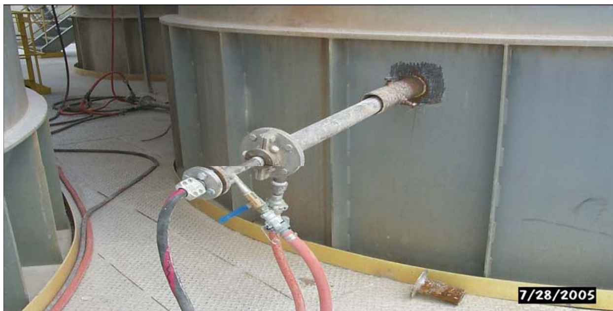
Figure 4-1.3. Application of SNCR at Holcim
