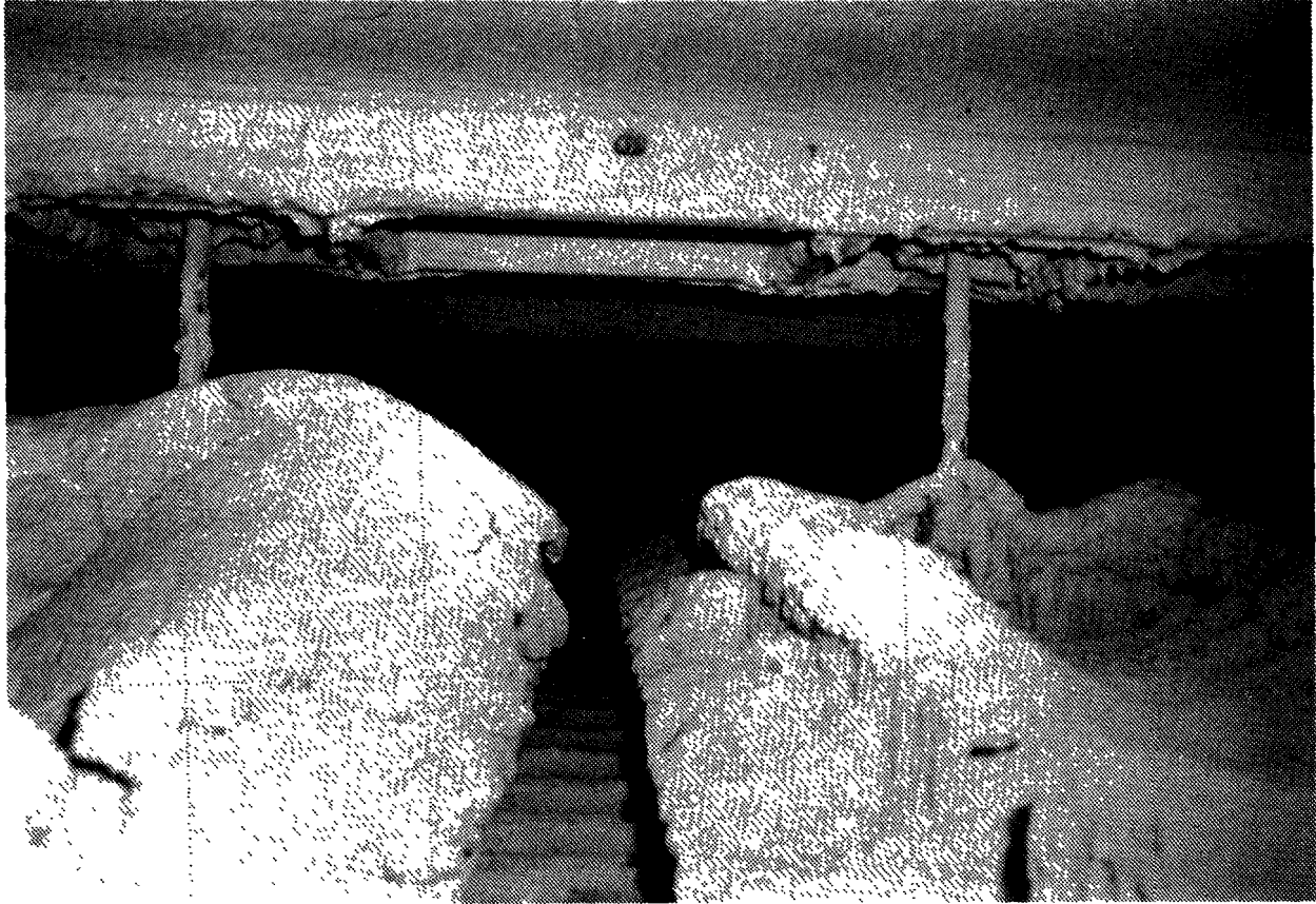
Figure 6-11. Accumulation of dust on rapper header beams.
